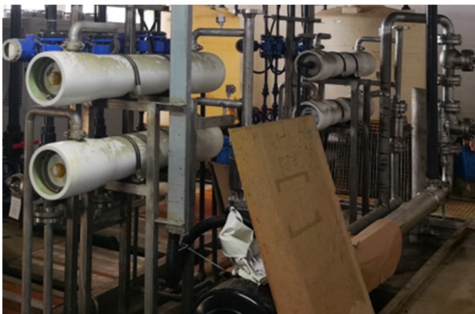
Figure 2. 8040 high-pressure membrane separation unit.
