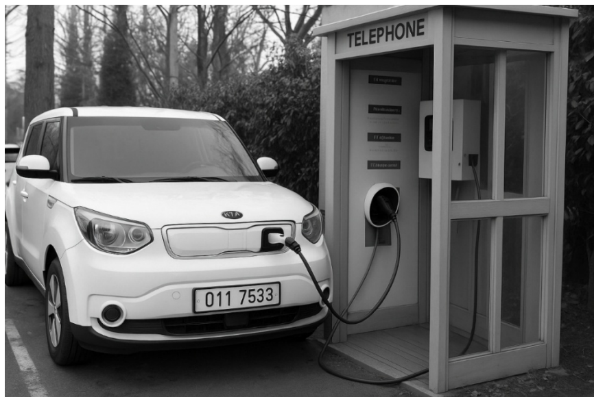
Figure 7. Charging station using a public telephone booth.
